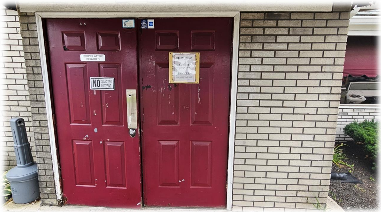
Door to be replaced in kind
